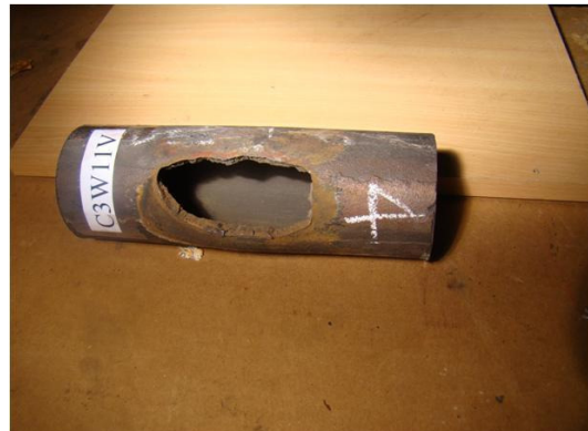
Fig. 23. A 'window' type rupture due to hydrogen damage in a waterwall tube.
